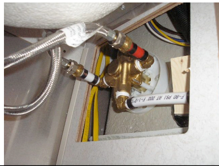
Supply at shower fixture
