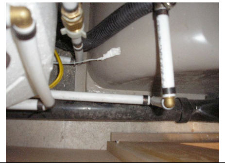
Coat hanger used to fish washer hose under water heater that is under the bathroom sink.
