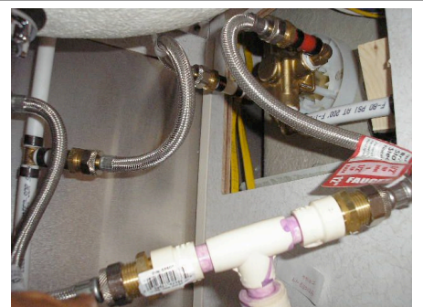
Tee installed in shower hot water supply line
